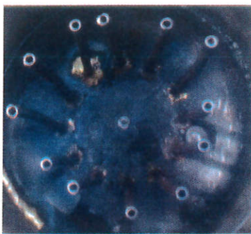
Plate 3.2 show the flanges in the water drum
