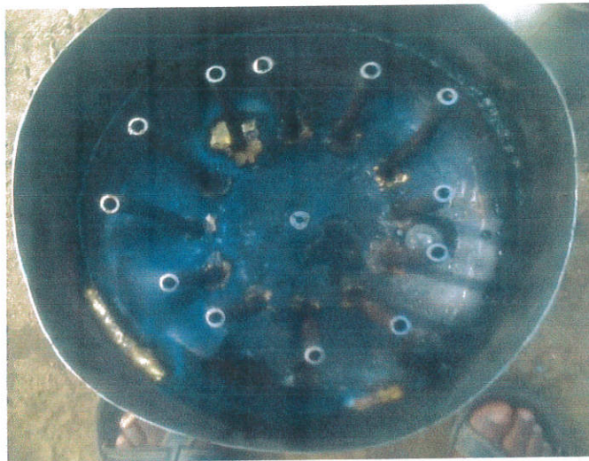
Plate 3.1 the steam section of the boiler
